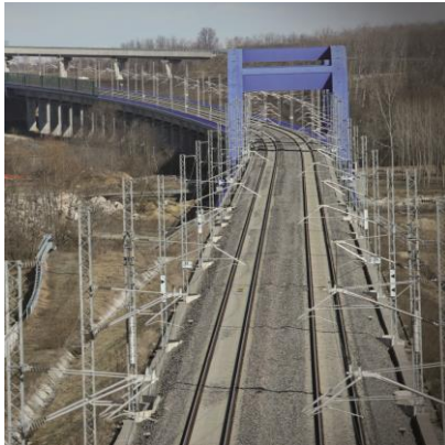
Construction of infrastructure works in preparation for Turin-Milan High Speed railway line (total length 36 Km)
